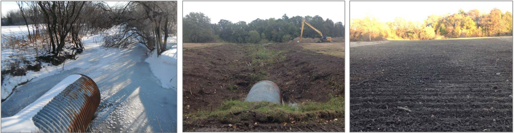
Figure 19 East pond outlet. Previous state (left), in progress (center), and after renovation (right) (facing South).
