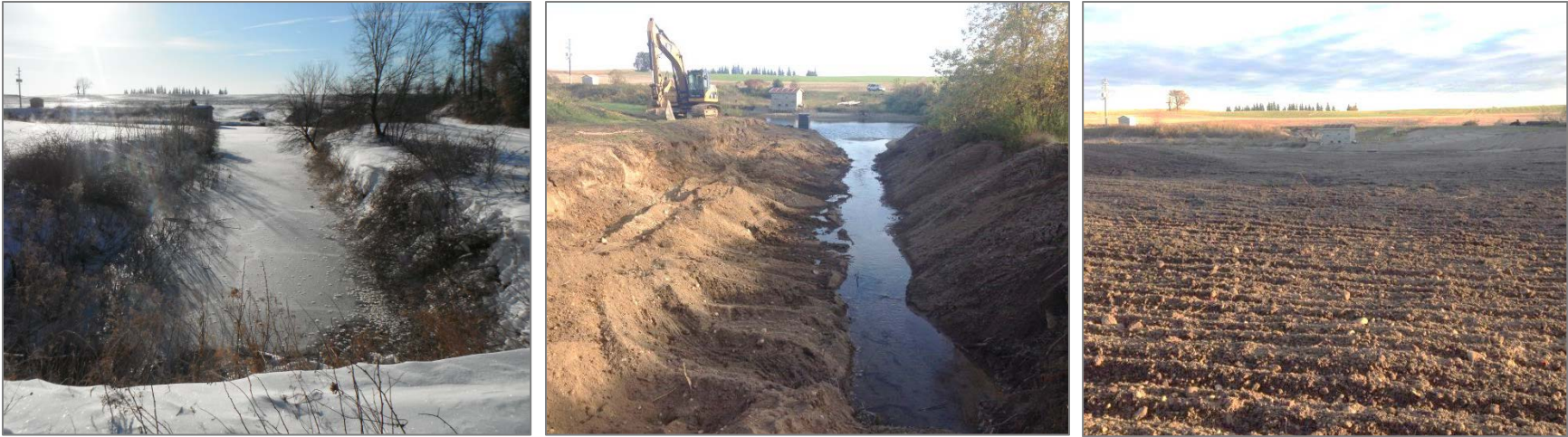
Figure 18 West pond outlet. Previous state (left), in progress (center), and after renovation (right) (facing South).
