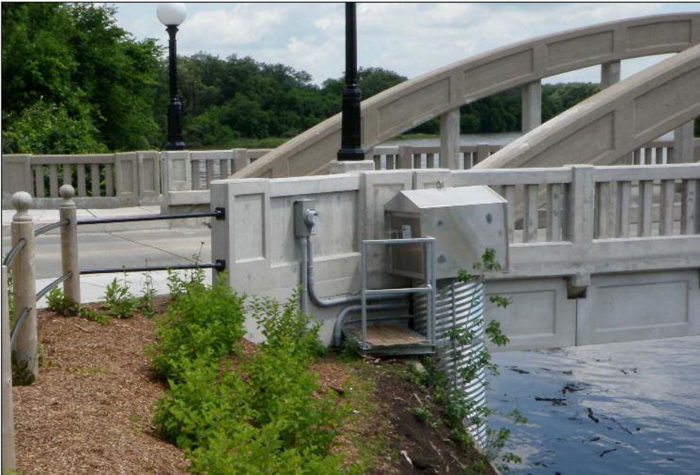
This flow gauge, located at Bridgeport Road in Kitchener, is one of 55 GRCA flow gauges used for flood forecasting and warning.
