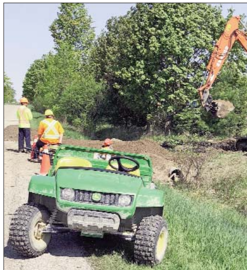
Students from Conestoga College build the road access, parking lot and school bus turning circle for the new Guelph Lake Nature Centre.
